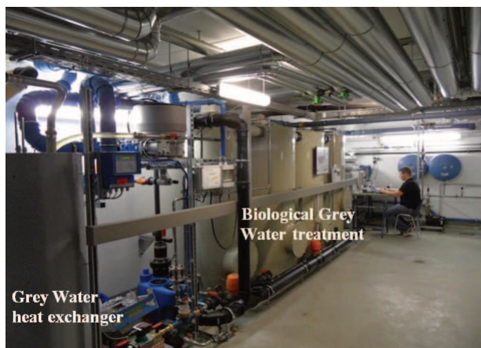
Fig. 7: Heat exchange and biological treatment of separated Grey Water in an apartment house in Berlin (Germany). Foto: H. Lehn
