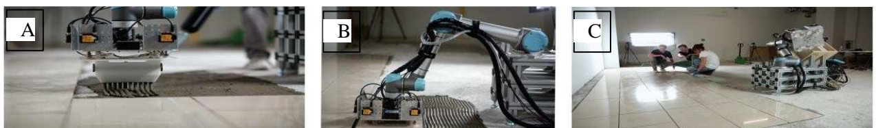
Fig. 22: tiles setting system A) mortar placement, B) tile placement; C) overview of the machine showing tiles placed (FCL, 2016).
