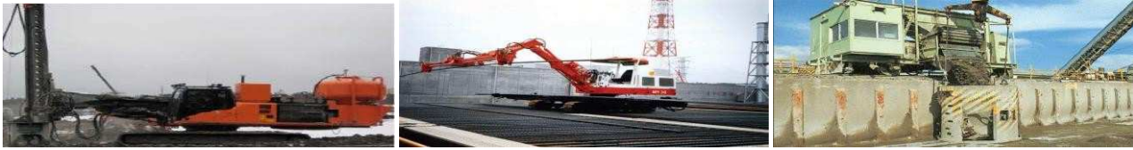
Fig. 5 (left): Pile driving machine (Hovila, 2012). Fig. 6 (middle): Reinforcement placing robot (Kajima, 2016). Fig. 7 (right): concrete distributor (Kajima, 2016).
