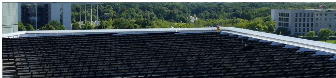
Fig. 12: Photovoltaics at Futurium, Berlin. © G.F.M. Baganz
