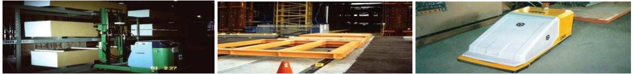
Fig. 16 (left): Material handling system (Obayashi, 2016). Fig. 17 (middle): Rail-guided system (Kajima, 2016). Fig. 18 (right): Automated mini- logistics unit (Takenaka, 2016).
